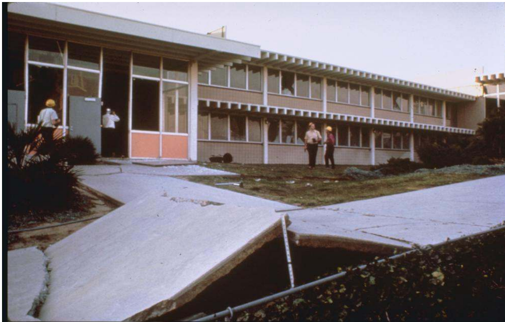
San Fernando Valley Juvenile Hall damaged by a 1971 earthquake. (Photo courtesy U.S. Geological Survey, credit E.V. Leyendecker.)
