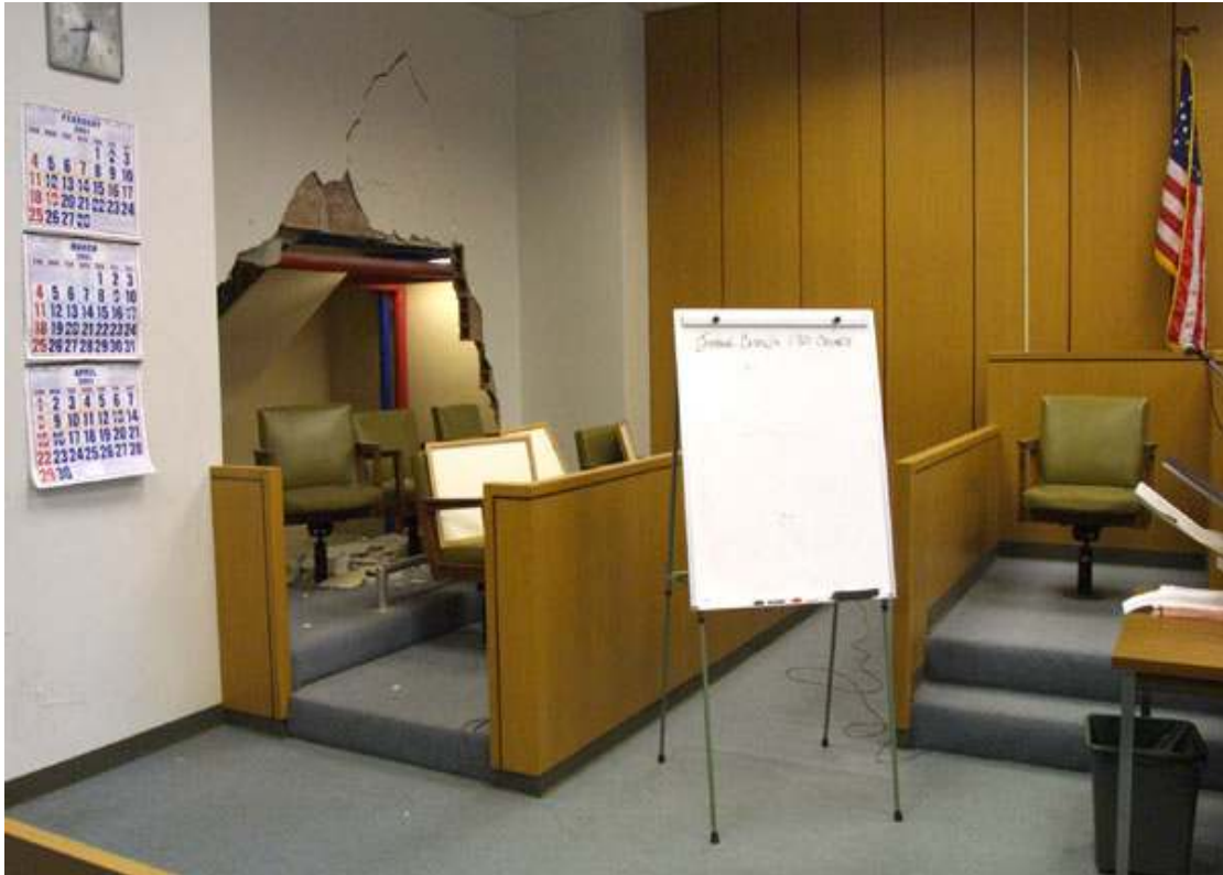
Damaged courtroom, King County, Washington Nisqually earthquake, February 28, 2001. (Photo courtesy King County, Washington State.)
